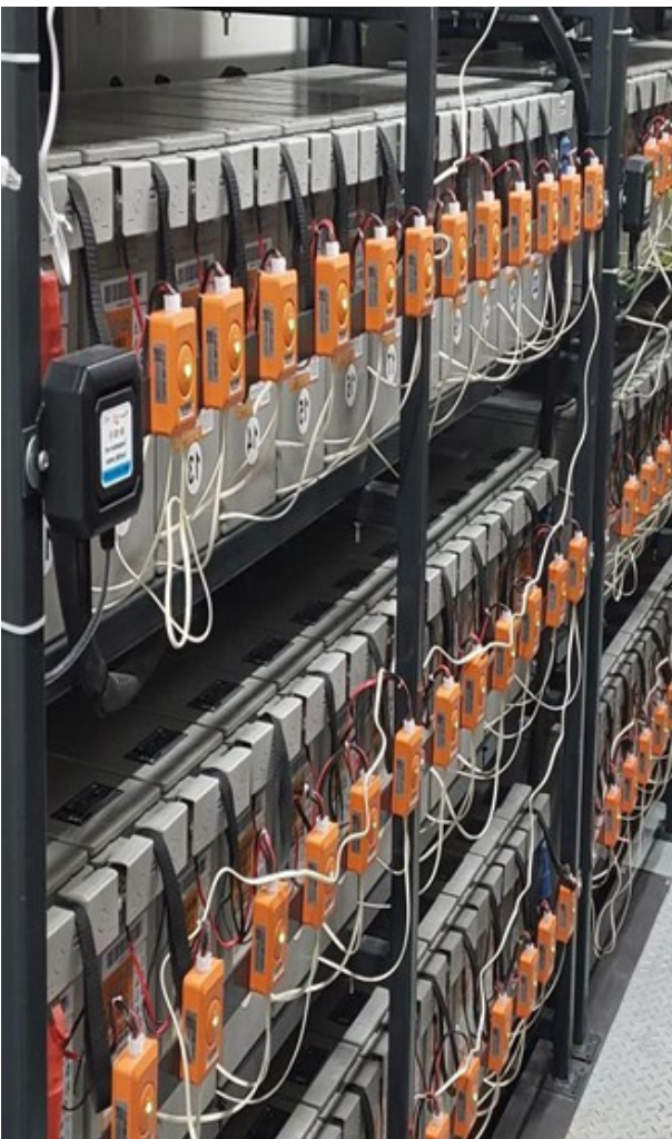
Reference project, GHD | Abu Dhabi, Implementiran BTMS
